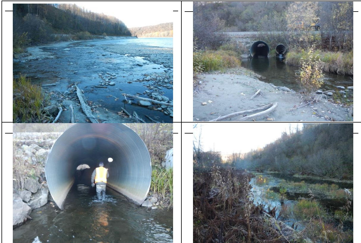
Figure 5.4-1. Photos of Lower McKenzie Creek/Slough, September 30, 2014. Clockwise from upper left: bottom of creek mouth; upstream view to culvert; culvert and beaver dam; and beaver dam above culvert and upstream of Alaska Railroad tracks.
