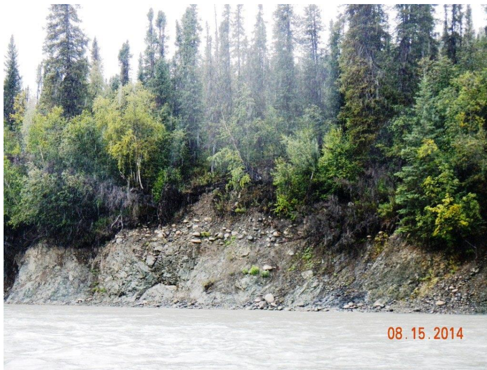
Figure A.2-77 - Susitna River right bank at PRM 202.7. Ice line on vegetation present in addition to eroded bedrock and outwash material (P250).
