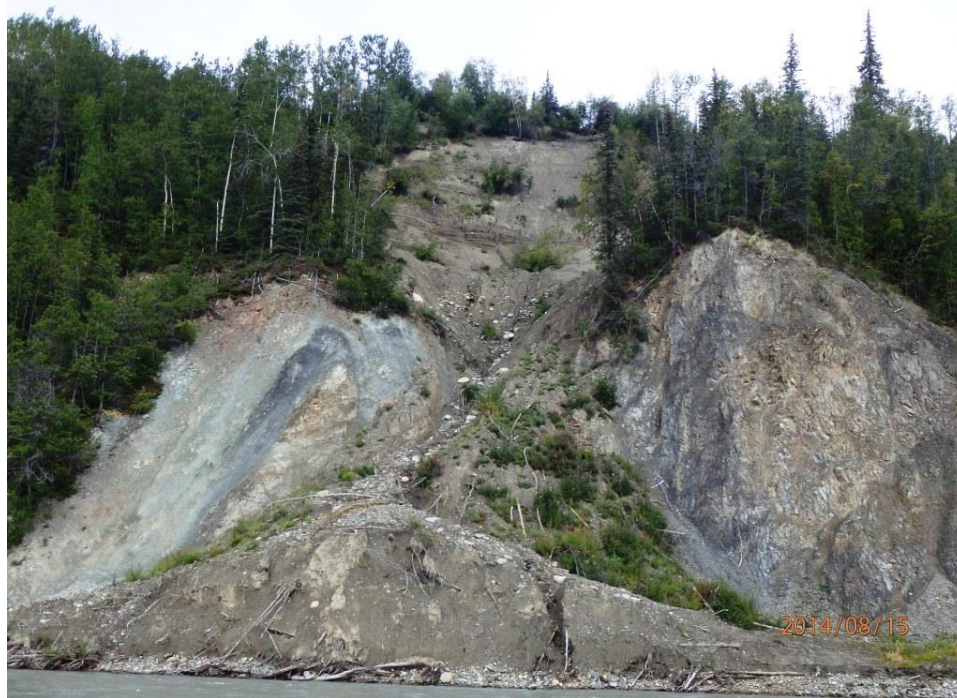
Figure A.2-64 – Active landslide zone on bend near PRM 209 – till over bedrock (P371).
