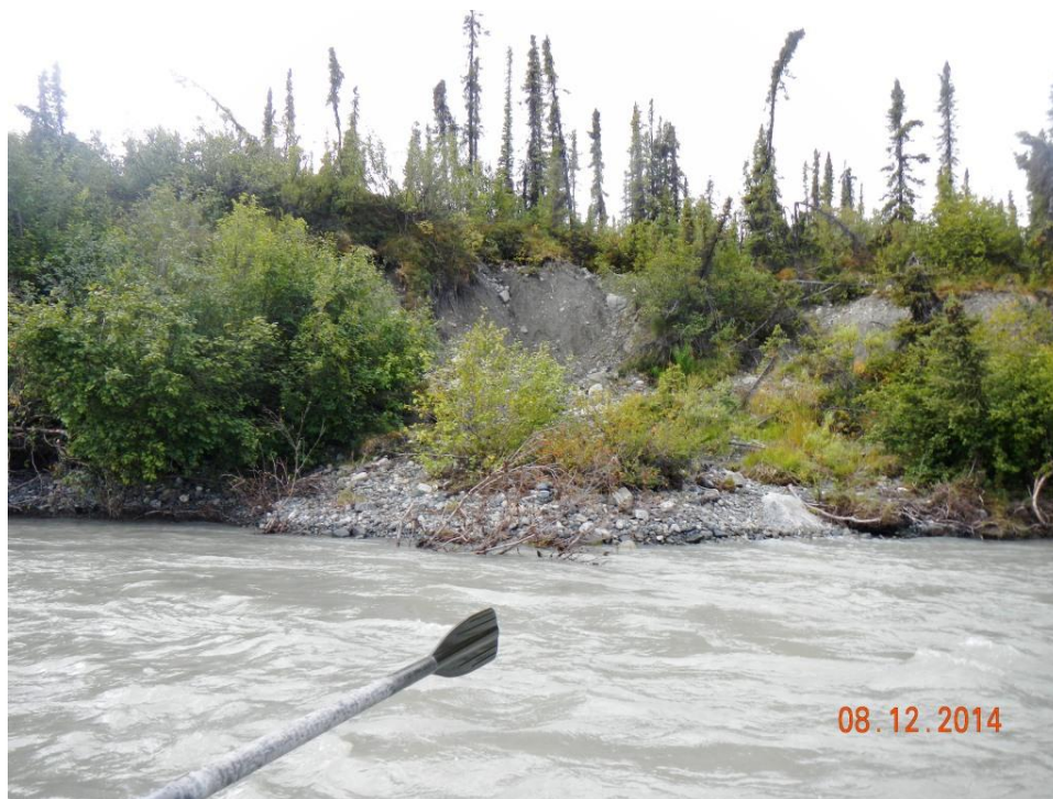
Figure A.2-31 – Pop out slide in till – local gravel source near PRM 240 (P554).
