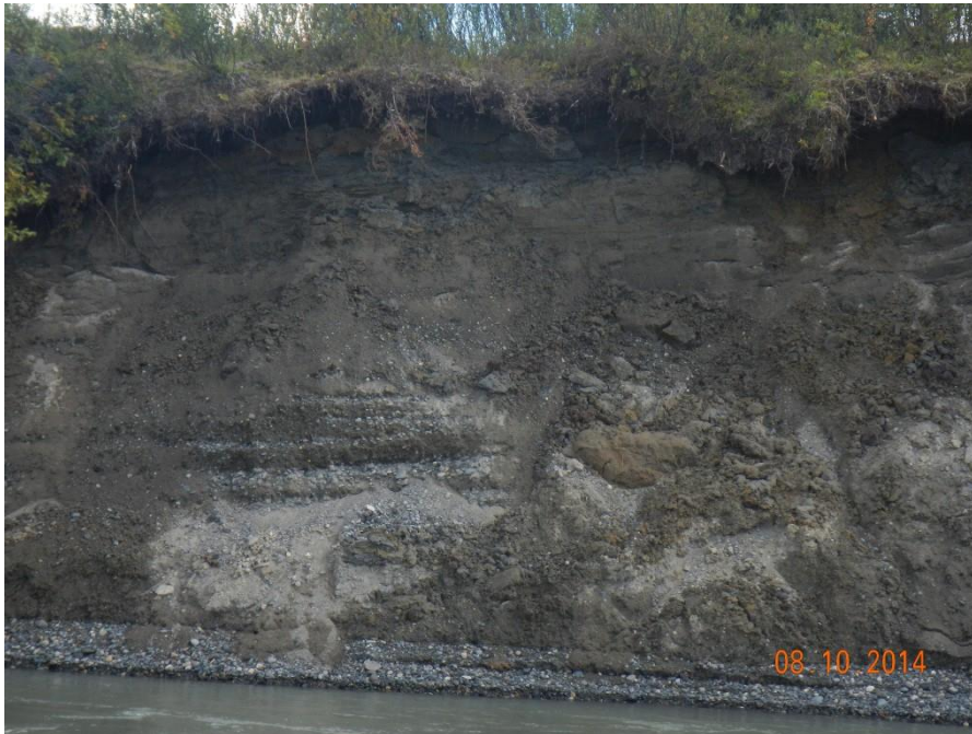
Figure A.2-2 – Eroding outwash terrace near PRM 260 (P213).
