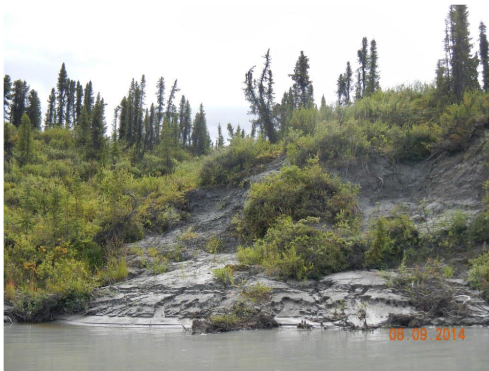
Figure A.1-14 – Active landslide in till near PRM 276. Failure may be due to melting of permafrost (P937).
