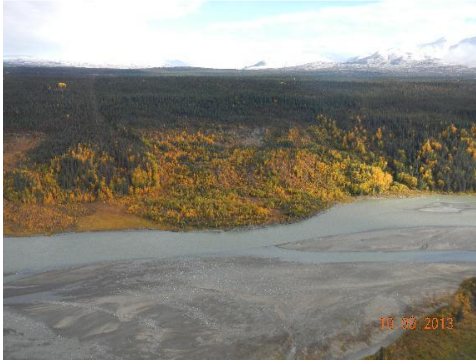
Figure A.2-80 – Active Landslide in till near PRM 200 – Susitna River right bank (P5459).
