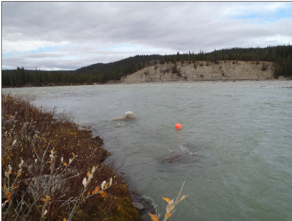
Photo A-37c. 2012 Buoy System Installed at PRM 235.2 – Oshetna Creek
