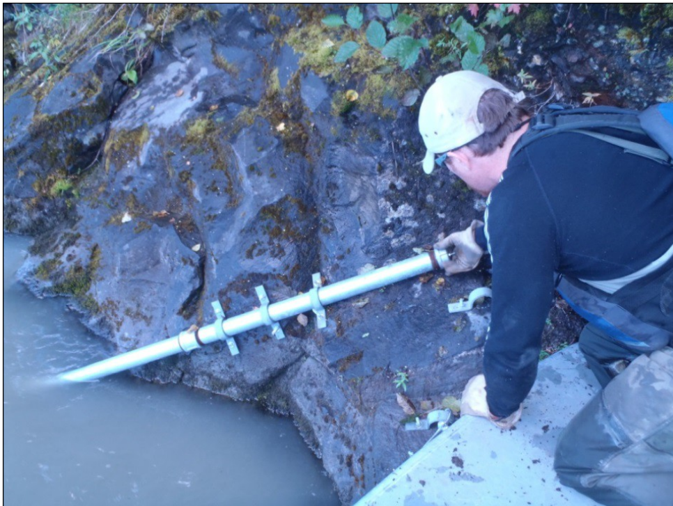
Photo A-23c. PRM 142.3 – Pipe mounted system at Susitna above Indian Creek
