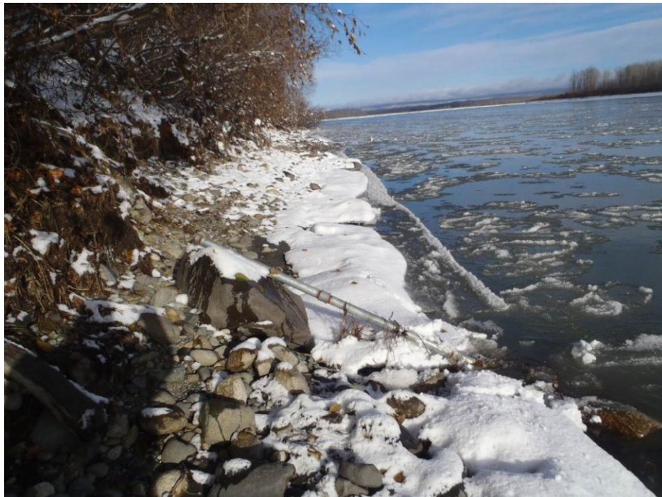
Photo A-8c. Pipe System at PRM 88.3 – Susitna at Parks Highway West
