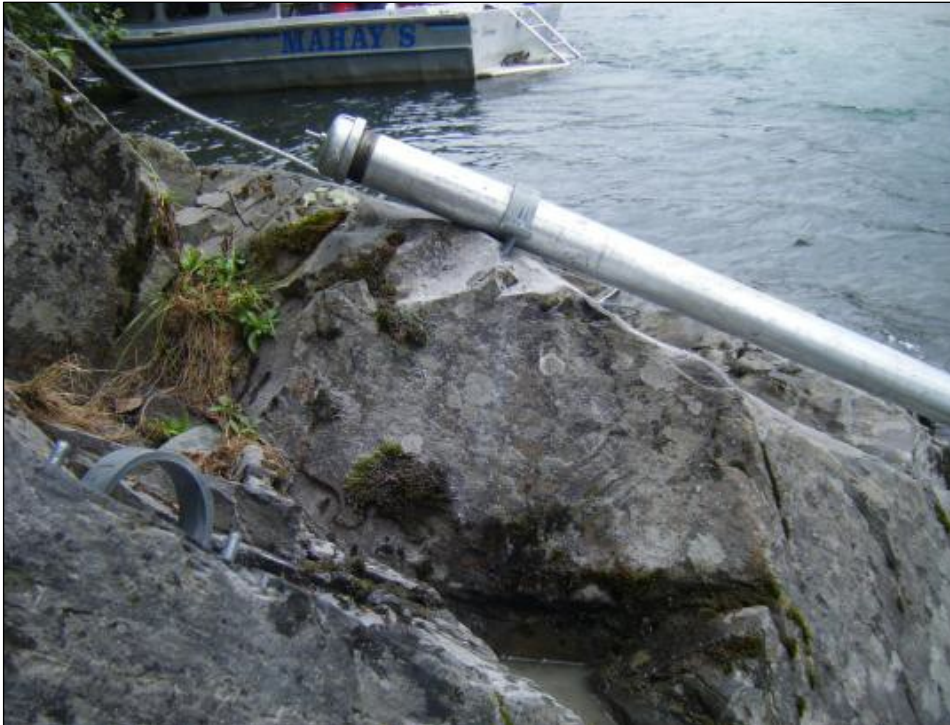
Photo A-27c. Pipe system at PRM 152.2 – Susitna below Portage Creek
