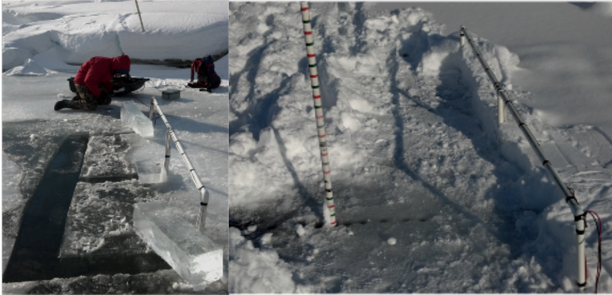
Figure C4.2-1. Swim-through test antenna installation through ice (L) and read distance testing following re-freeze (R).
