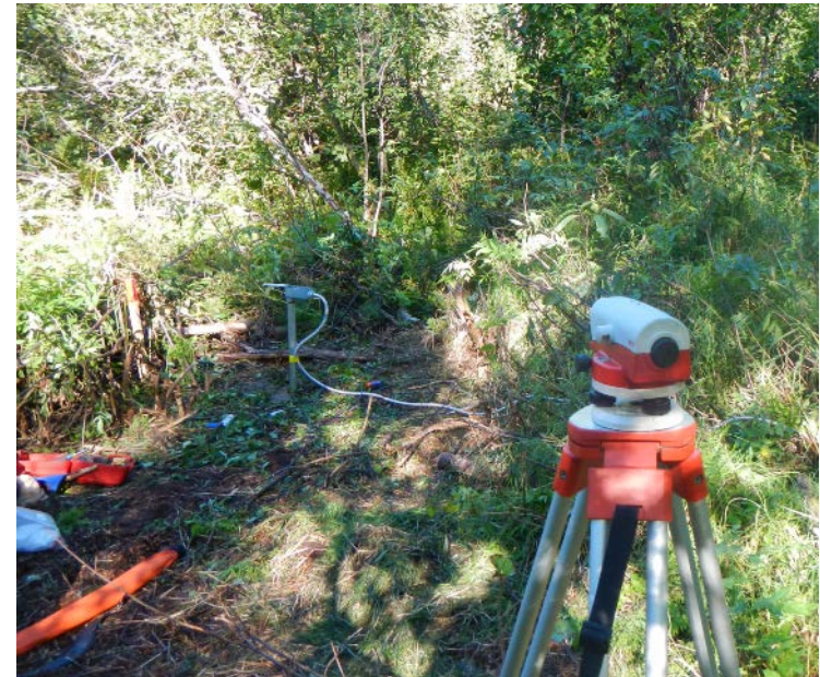
FA104 – Whiskers Slough - surveying a new well installation to measure water levels to Project datum and accuracy standards, August 27, 2013
