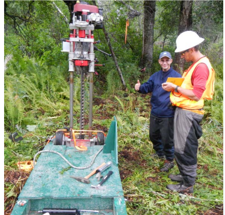
Portable drill and custom sling-load cradle/sled at FA104 – Whiskers Slough after another successful boring completion, August 24, 2013
