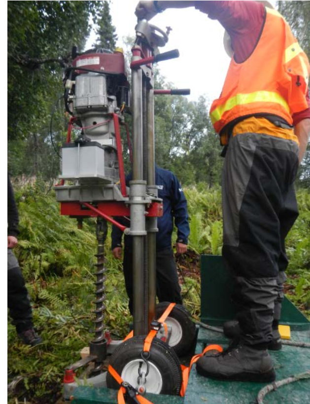
Mobile Drill Minuteman portable drill being used to pre-drill drive point well installation borings, drill is sitting on custom sling-load cradle, August 23, 2013
