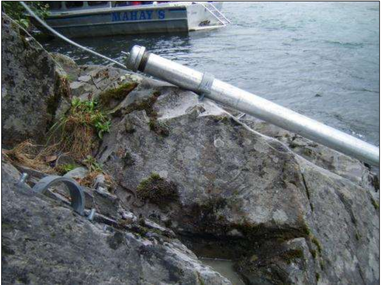
Pipe System at RM 148.0 – Susitna below Portage Creek
