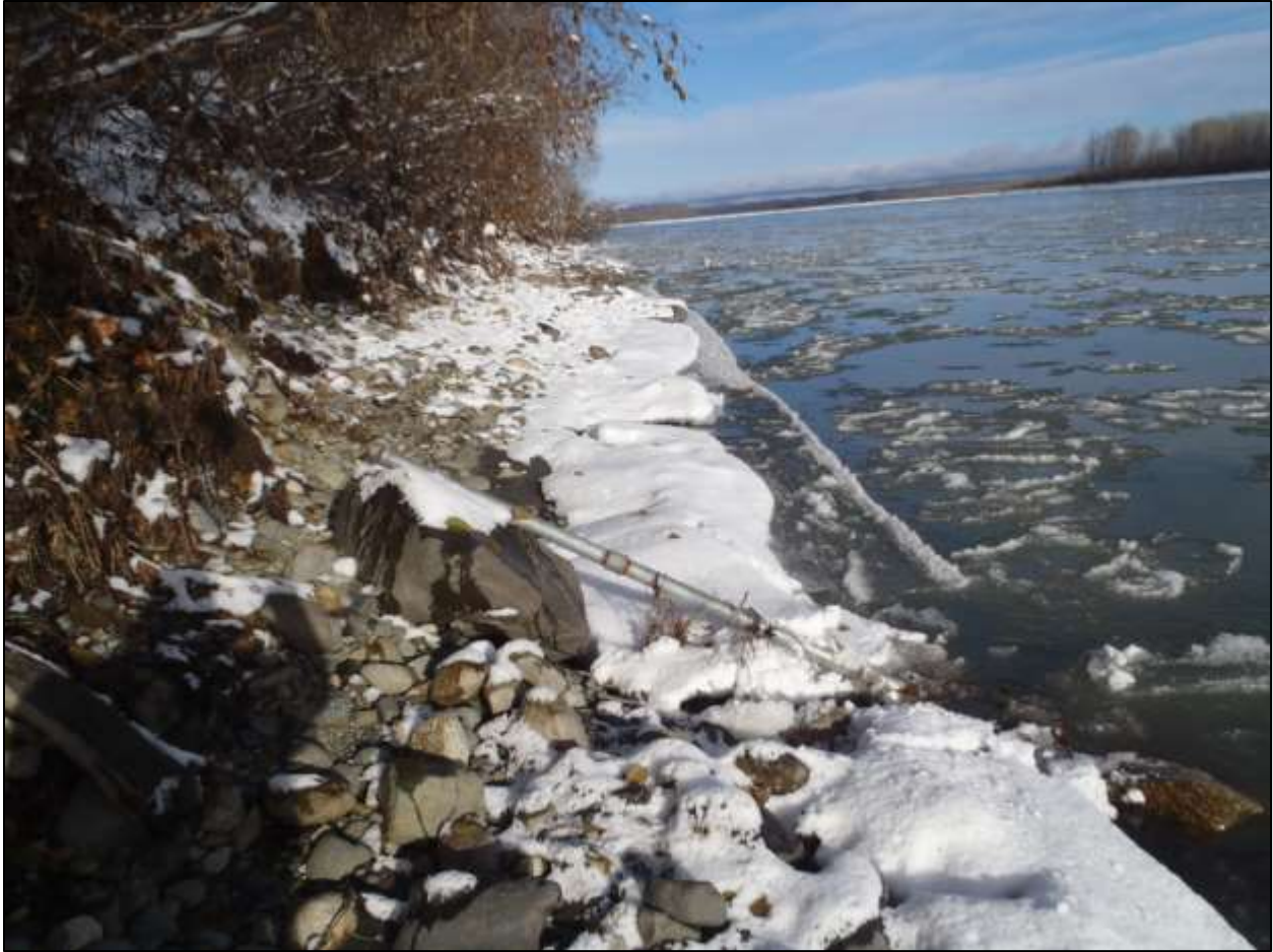
Pipe System at RM 83.9- Susitna at Parks Highway West
