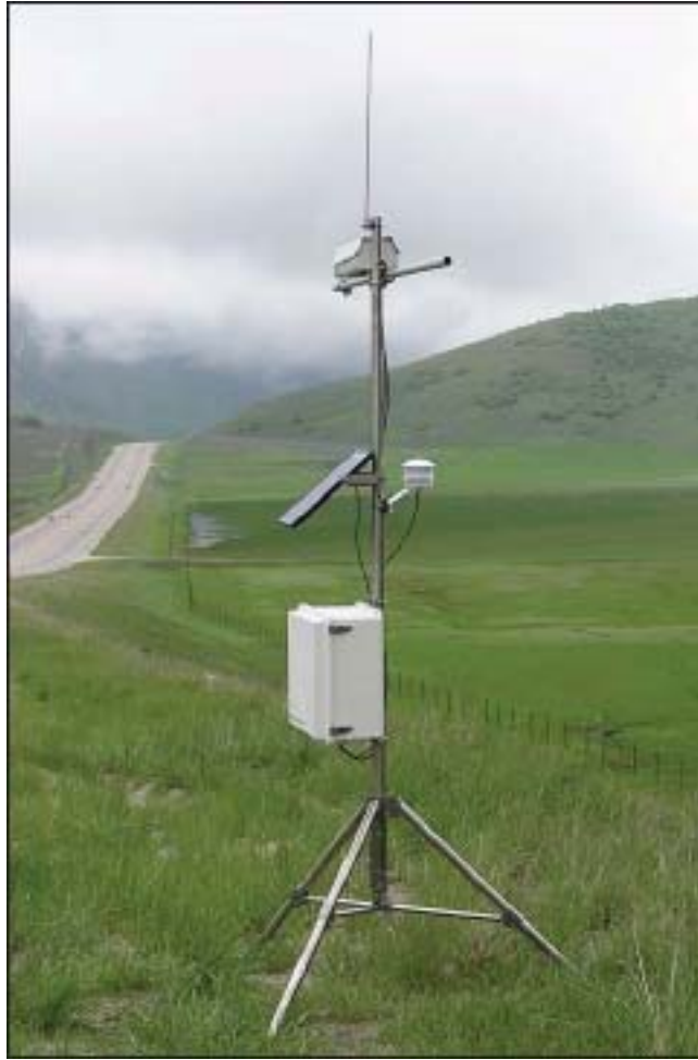
Figure 5.5-2. Example of a 10-foot (3-meter) tripod MET station (guy wires for stabilization and an enclosure will be installed).
