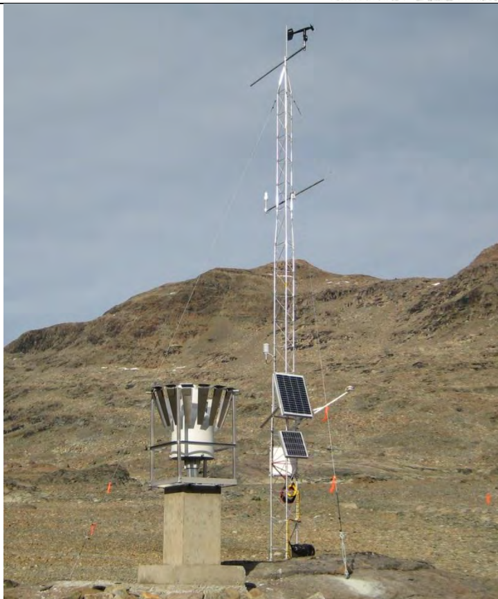
Figure 3. Example Meteorological Station Installation
